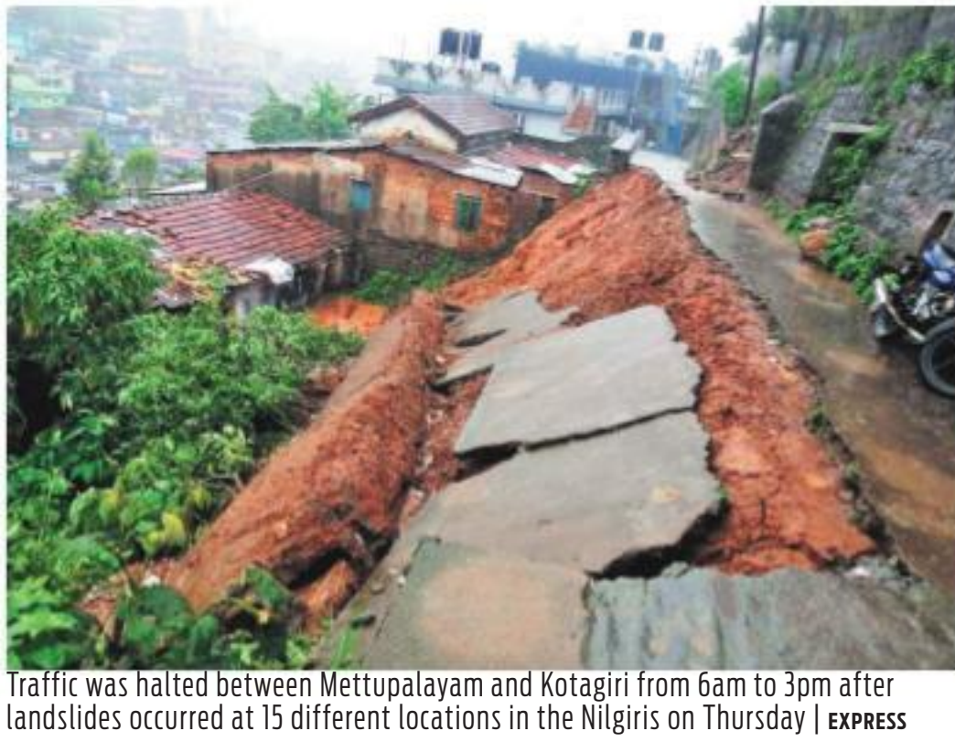
Traffic was halted between Mettupalayam and Kotagiri from 6am to 3pm after landslides occurred at 15 different locations in the Nilgiris on Thursday | EXPRESS
